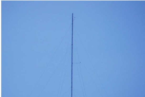
Missing 30 m anemometers, Feb 2010; D. Vaught photo
