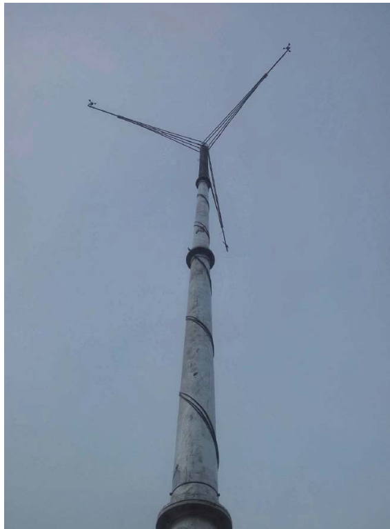
Tower sensor photograph, south side (Marsh Creek, LLC photo)
